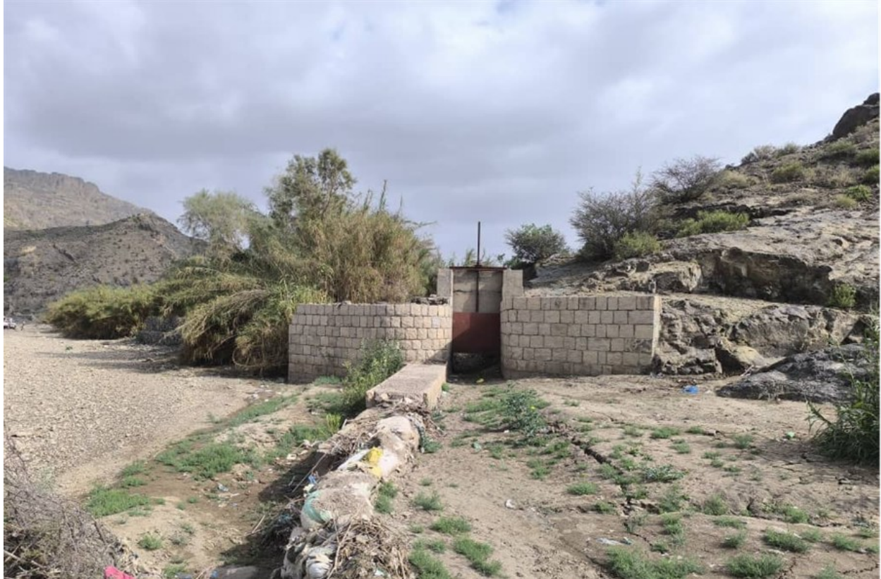
An irrigation canal that has gone out of service in Al-Mosaymer district. | Photo credit: UNDP.
